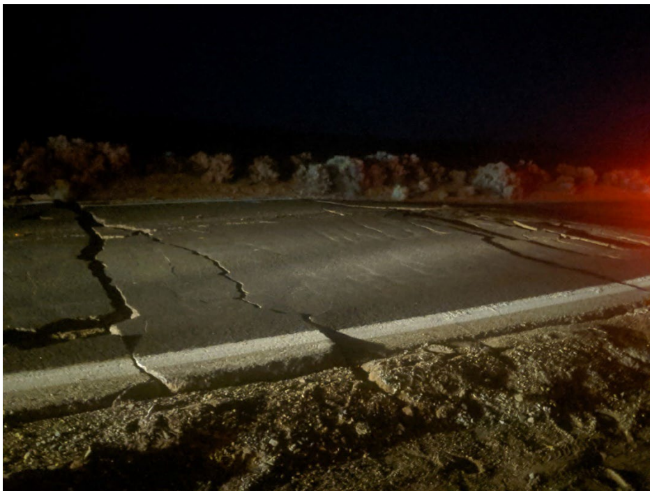
Surface rupture of M7.1 taken hours after the rupture along Highway 178 (July 5, 2019).
